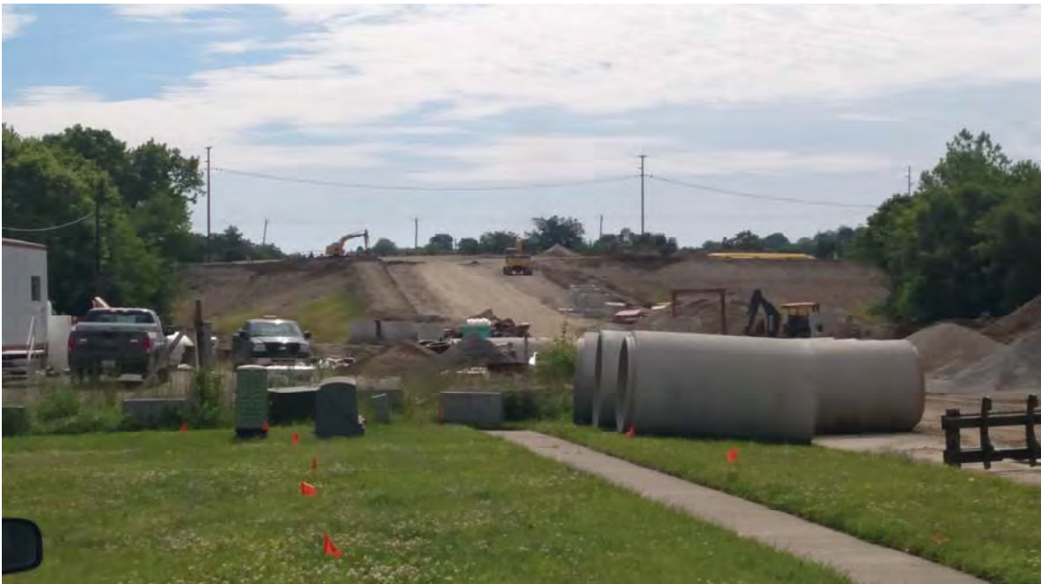
South Hamilton Crossing with the new MSE wall where the new overpass at the railroad crossing will be constructed (top). The western end that is being built up to accommodate the increased height of the road (bottom.)
