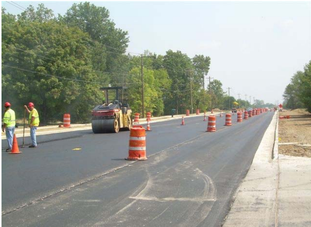
Western Row Road improvements will enhance a major east-west route in the city.
