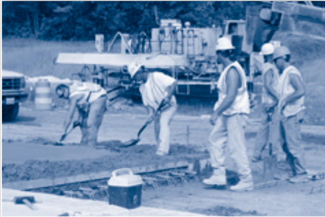
Construction crews begin grading the area so paving can begin at Interchange #140 (State Route 58).
