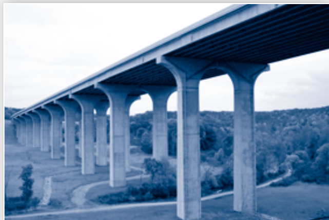
The Cuyahoga River Bridges span 2,682 feet above the Cuyahoga Valley National Park in Summit County.
