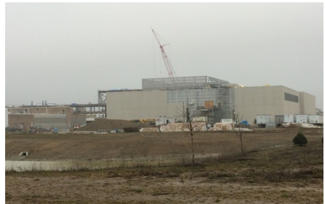
P&G Beauty Innovation Center continues construction at its existing business center 241-acre campus on Mason-Montgomery Road. The 500,000 square foot project is making timely headway and expected meet its completion date of early 2019.
