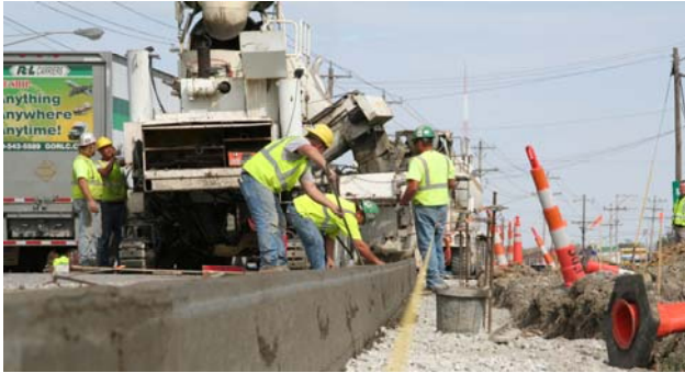
Improvements on U.S. 42 from Tylersville Road to Butler-Warren Road began in 2011 and will be complete in 2012
